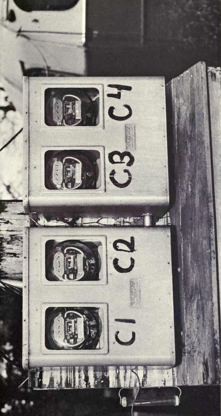
PLATE 9.—Illustration shows typical electric-meter-box installation
