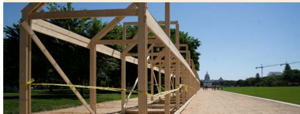
Installation of HUD's Innovative Housing Showcase on the Mall Copyright Victoria Pickering, Flickr
